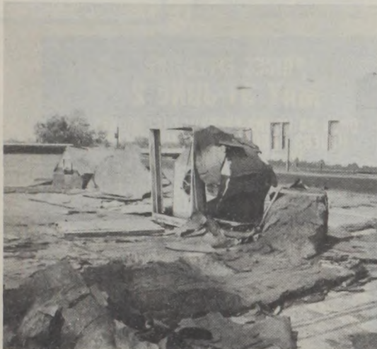
This picture was taken of the roof at City Drug showing extensive damage to the roof, the skylight and the air conditioner.
