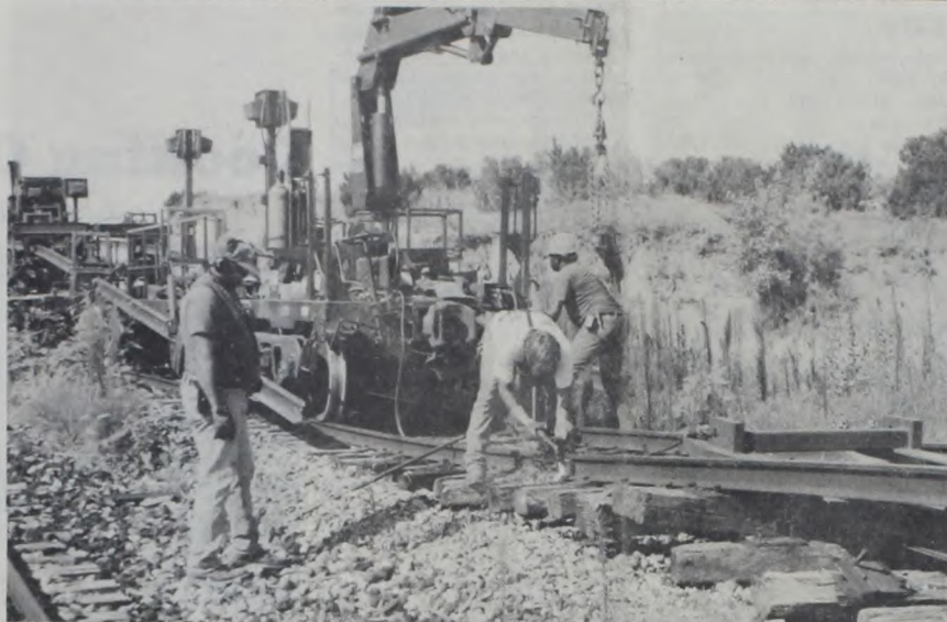
Trent McKay (white shirt) and unidentified hands of Burlington-Northern railroad work crew, begin tearing out the rails to the tunnel. This view is looking south from the Los Lingos river railroad bridge.
