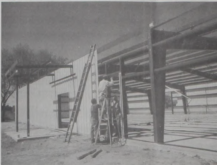
Quitaque's new Community Center is quickly becoming a reality. Area residents are excited about the new multi-purpose facility that will soon be available for use.
