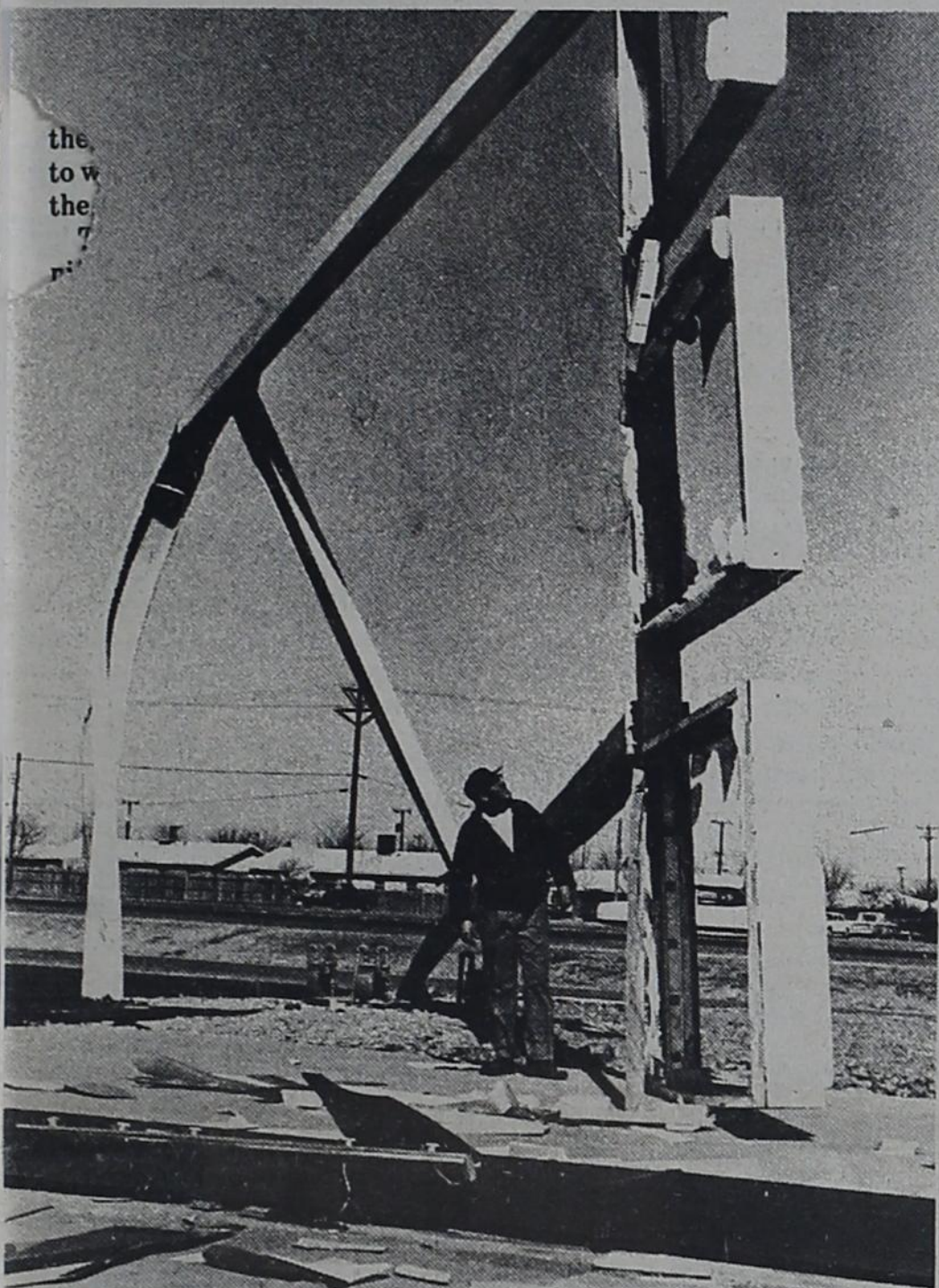
WIND DAMAGE LAST THURSDAY—Frank Henry, operator of Frank's Fina in Wolfforth, is shown examining the twisted remains of his 65 foot Fina sign that was destroyed last Thursday afternoon by the high winds. The sign toppled at about 5 minutes after 2:00 and fell in the middle of a new building site next to the Fina station. Fortunately, only the foundation and floor had been poured for the new building. (Staff Photo)
