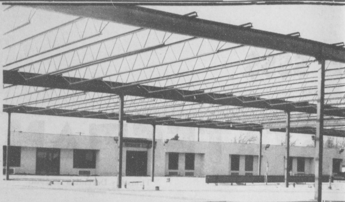
Work is progressing on Hansford Manor. The steel was erected during the Thanksgiving week. Because of the beautiful weather work is progressing on schedule at the Manor. Drive by and look at the Manor today.
