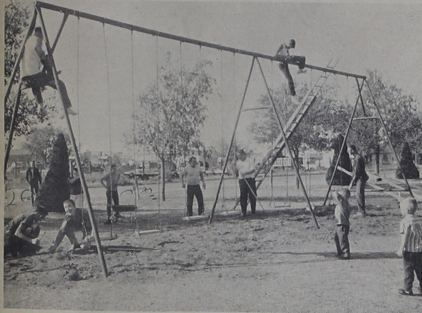
The Boy Scouts were hard at work repairing the swings and see-saws in the Gruver Park on Sunday. This is a project undertaken by the boys. They will paint the swings at a later date.
