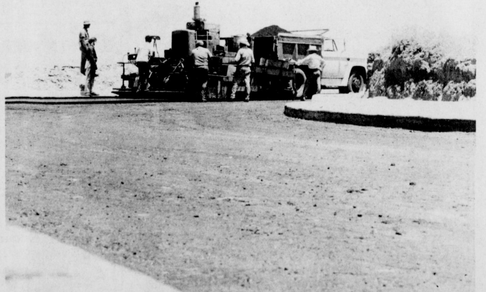
PAVING PROGRESSES near the high school building in the west part of town, and likely will be completed by the end of this week. The workmen are shown laying asphalt on the south access road by the expressway Tuesday. Another road is currently under construction near there. Edgell Trail in Park Plaza was opened this week. Several new houses are planned for the new area.
