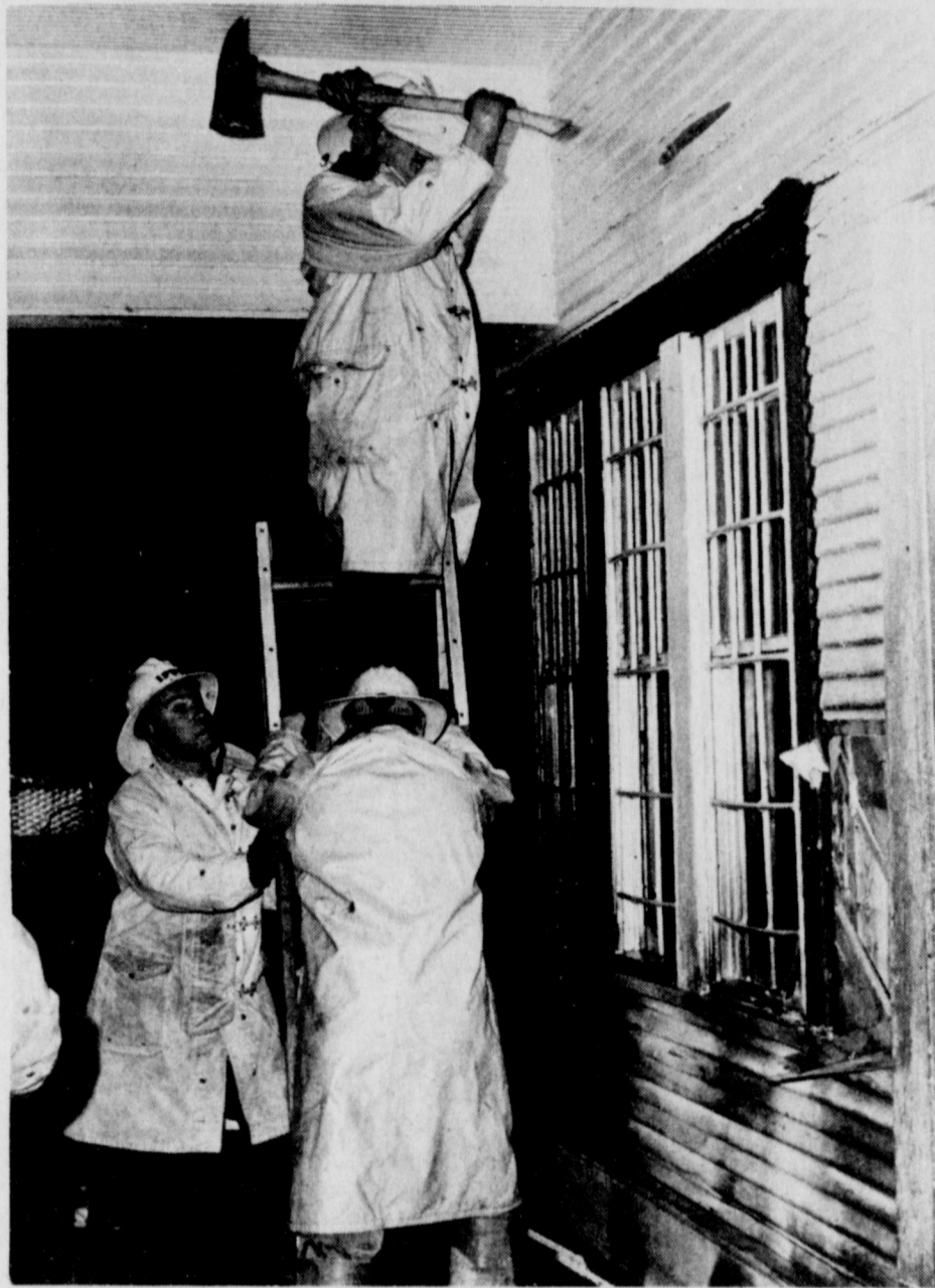
FIREMEN had to use an axe to reach the interior of the double wood wall before extinguishing flames at Sisk Bullets Monday night.
