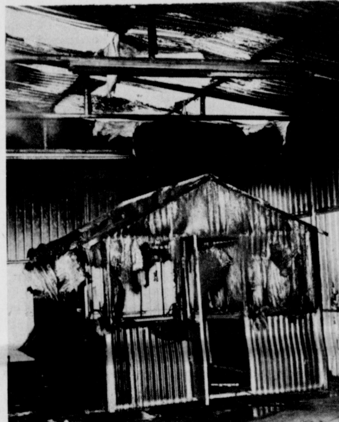
FIRE DAMAGE - A metal building and a smaller structure inside were heavily damaged Saturday afternoon in a flash fire. Ricky Vanek was reportedly welding in the building when heat apparently ignited some flammable materials. No one was injured, according to reports. The structure, owned by Bill Vanek, is located on the east side of Gilmore Welding on Highway 287.
