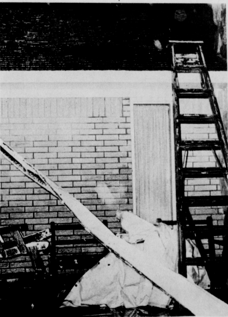
ROOF DAMAGED by sailing metal at Harold Cowley home, 505 W. Rebecca.
