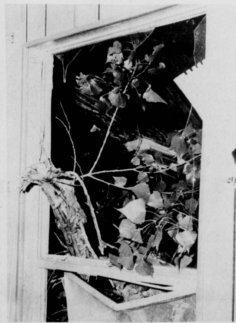
BROKEN LIMBS invade mobile home at Valley View.
