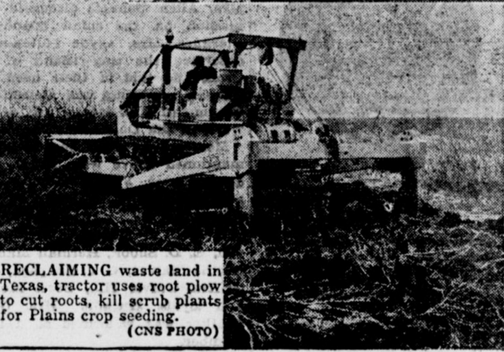
RECLAIMING waste land in Texas , tractor uses root plow to cut roots, kill scrub plants for Plains crop seeding. (CNS PHOTO)
