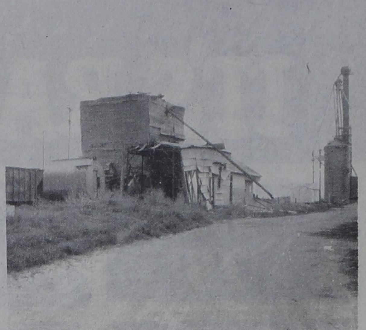
A PORTION of the old Farmers Elevator in Munday, operated by the late M. H. (Marvin) Reeves for many years, was toppled by high winds recently, blocking a portion of the Burlington Lines railway track. Workers were busy clearing the track last Monday.
