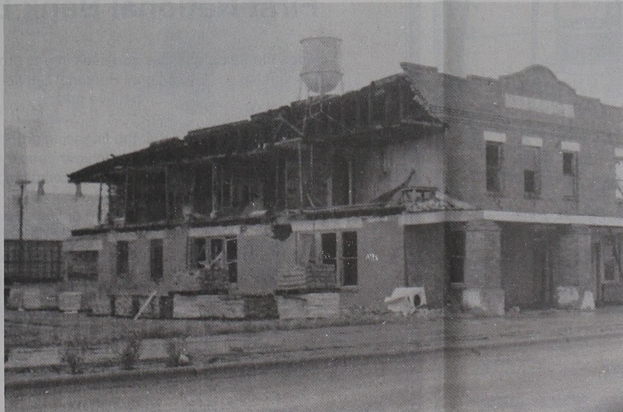
THE WALLS ARE COMING DOWN. The Munday Hotel building was constructed before 1920 and in use until the late 1950's. Today the structure is no longer of any use and had become an eyesore. Farmer's Grain Coop has purchased the property. Since the railroad will be shipping very little, if any, such coops will have to find other means of shipping which will be trucking. A road will be put on the property to keep congestion from building up around the grain elevator during wheat harvest.
