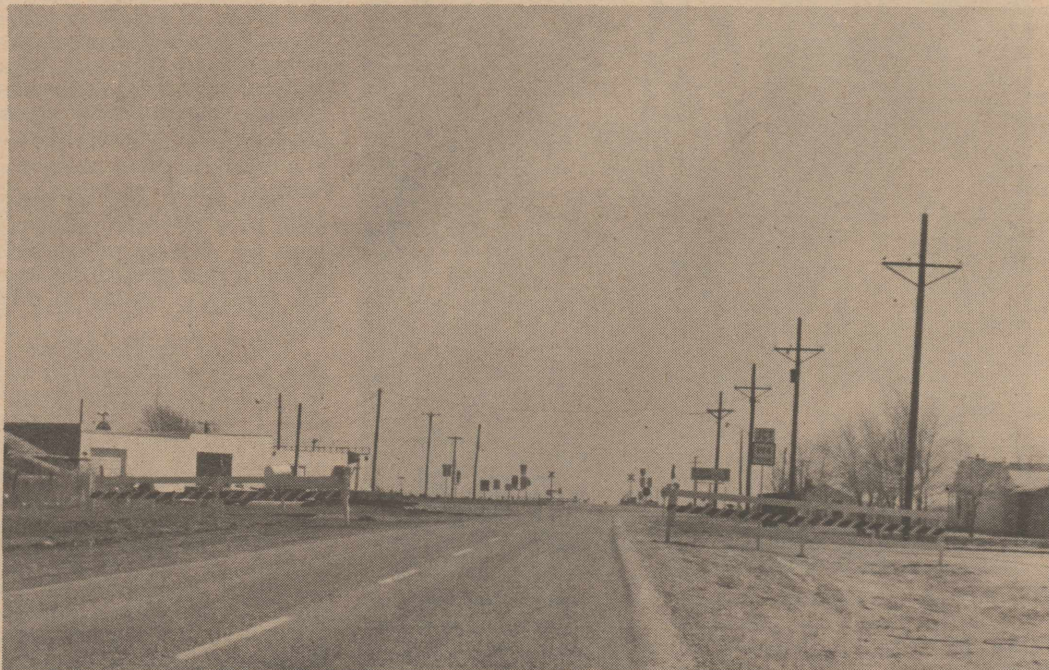
CONSTRUCTION BEGINS on the highway between Hart and Edmonson which will have a sealed shoulder along the old highway.
