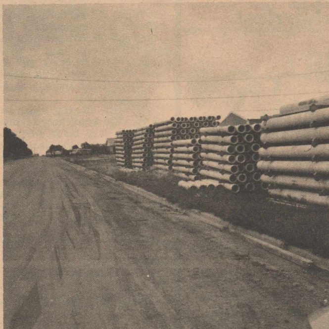
PIPE FOR NEW WATER LINES arrived this week in Hart. The new water lines will be laid in the south part of Hart, replacing the old small pipe line which runs there now. The residents in that part of town have been receiving about one third as much water as the rest of the town for the past several years. Drake & Clayton of Lubbock are the contractors in charge of the new lines.
