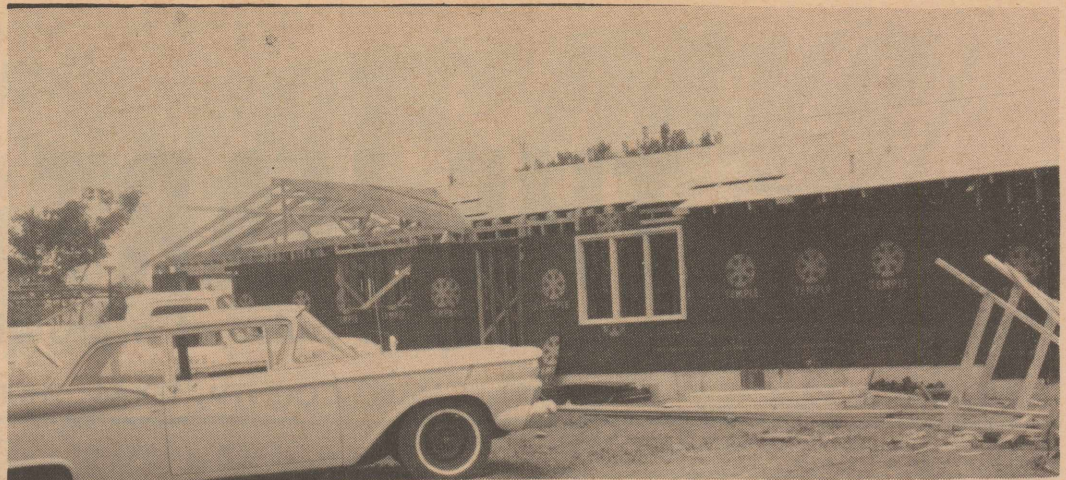
JUDD DAVIS HOME--Work is progressing on the new home of the Judd Davises, shown above.
