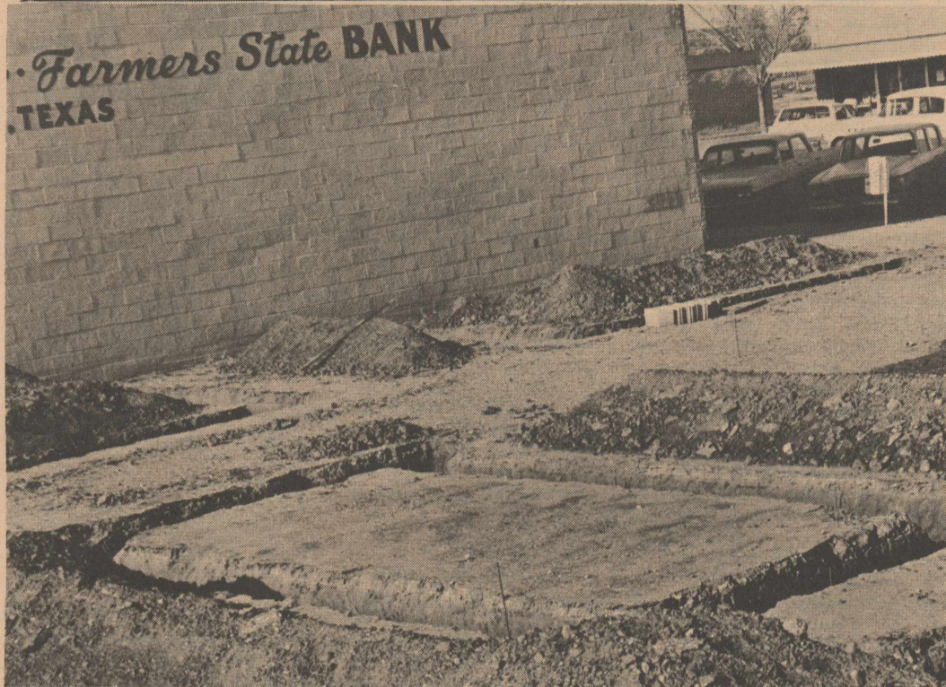
WORK STARTED last week on an addition to Farmers State Bank but rains stopped construction after foundation work was begun.
