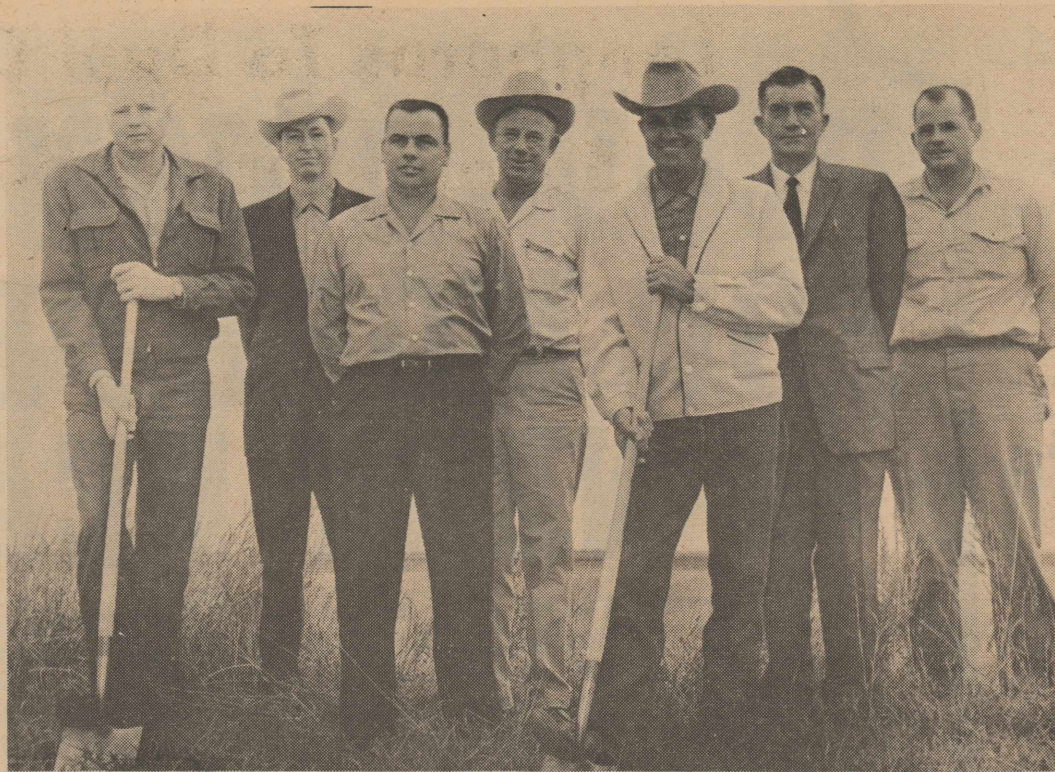
GROUNDBREAKING for a new high school and gymnasium got underway last week across the street from the present Hart school. School trustees were present and classes were turned out for the historic event. In the picture stairstepped from left to right are R. G. Henderson, board president; Chas. B. Martin, Doyle Davis, Lorenza Lee, Milton Sharp, secretary; Paul Kennedy, supt; and building contractor representative Ray Nixon.
