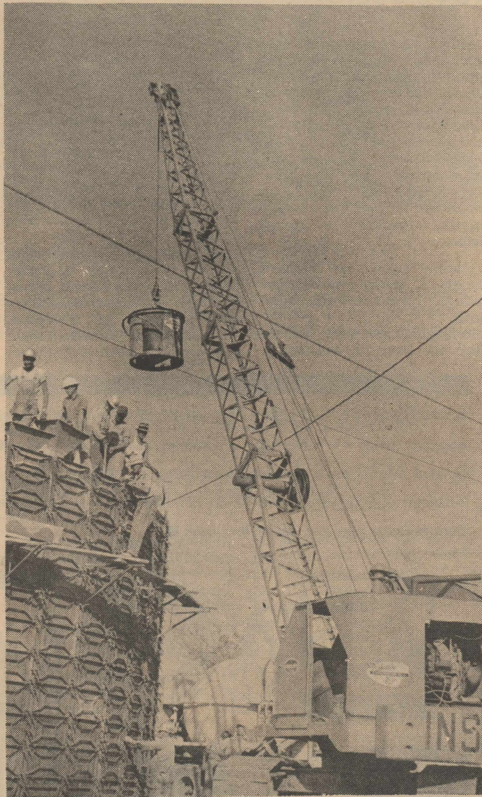
WORK Continues here on part of Hart's water and sewer project. The project will be completed near the end of this year. Besides a sewage lift station, construction of a network of sewage pipes continues at full speed.
