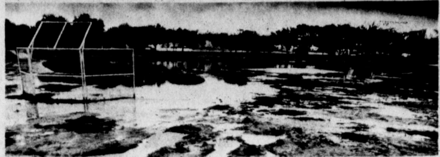
The five-acre Wadley-Barron Park in east central Midland will be more of a wavy lake than a grassy park by September, when work is to be completed on the proposed lake. The park is bordered by Cuthbert and Harvard avenues and by A and B streets. Excavation is to begin in mid-May. About 15 elms trees in the right background will be removed to make way for the enlarged pond.
