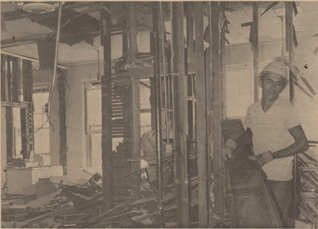
COURTHOUSE DEMOLITION—This picture was taken early this week in the second story of the hospital building, after workers began demolition of the building last week. Manager of the demolition project here said the building probably will be completely torn down in about two more weeks. Shown here is a view of the east wall.
