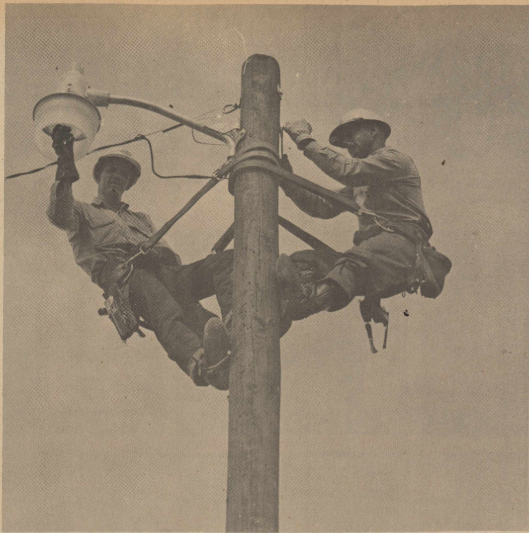
INSTALLING NEW LIGHT---Leonard Stamps, left, and Johnny Schenck, service men for Olton Southwestern Public Service, are shown installing a Guardian light at the Clifford Carlisle farm. It was the first light of this type to be installed in the Olton area. The 7,000 Lumen mercury vapor light comes on automatically at night and goes off in the day.
