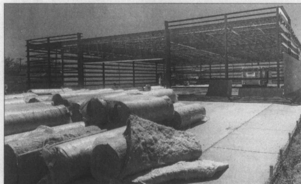
Future Family Dollar store ... Construction continues as the framework goes up on a new 9000 sq. ft. building for the new Family Dollar store in Tahoka, on property adjacent to the Cash Saver Supermarket on Lockwood. The space was formerly occupied by the LCHD Specialty Clinic, which was demolished when LCHD sold the property to the Family Dollar franchise.
