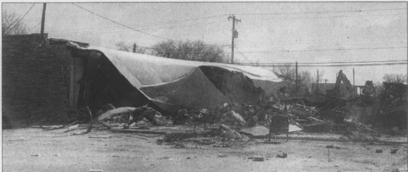
Future Family Dollar store ... Demolition began last week as the former LCHD Specialty Clinic was torn down, to make way for a new Family Dollar store. The Lynn County Hospital District sold the property that sits adjacent to the Cash Saver Supermarket on Lockwood in Tahoka, finalizing the sale a few weeks ago. The plans call for a 9000 sq. ft. building for the new Family Dollar store, according to Tahoka Mayor John Baker.
