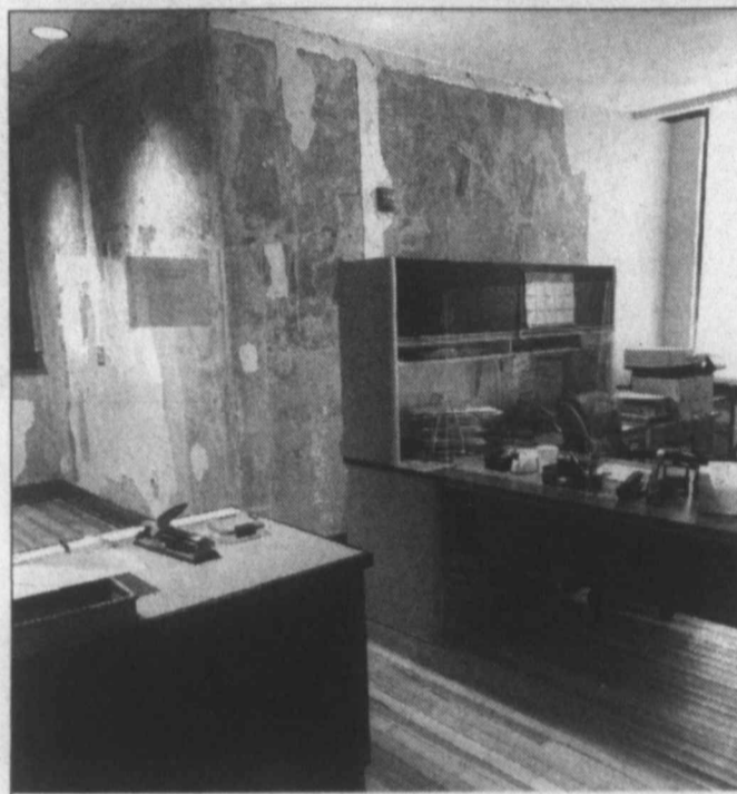
Walls damaged ... The Lynn County Clerk's Office on the first floor of the Lynn County Courthouse had extensive damage after the recent flooding mishap from a burst waterline connection. The walls, which in this photo look a little like a printed wallpaper, is actually mottled coloring from stripped plaster. In this office, ceilings, walls, and wood floors will all require replacement or repairs, and much of their office equipment was damaged from water as well. (LCN PHOTO by Juanell Jones)
