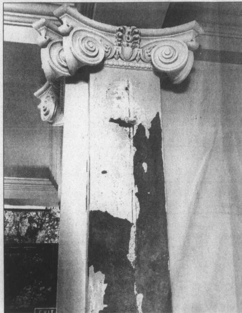
Courthouse foyer ... Water has damaged the plaster on the walls beneath the ornate scrolled cornices in the foyer at the first floor entries at the Lynn County Courthouse, but the historic scrolled cornice work appears to have survived any damages, after the recent flooding mishap that caused water to run down walls and ceiling from the third floor to the basement level of the courthouse. (LCN PHOTO by Juanell Jones)
