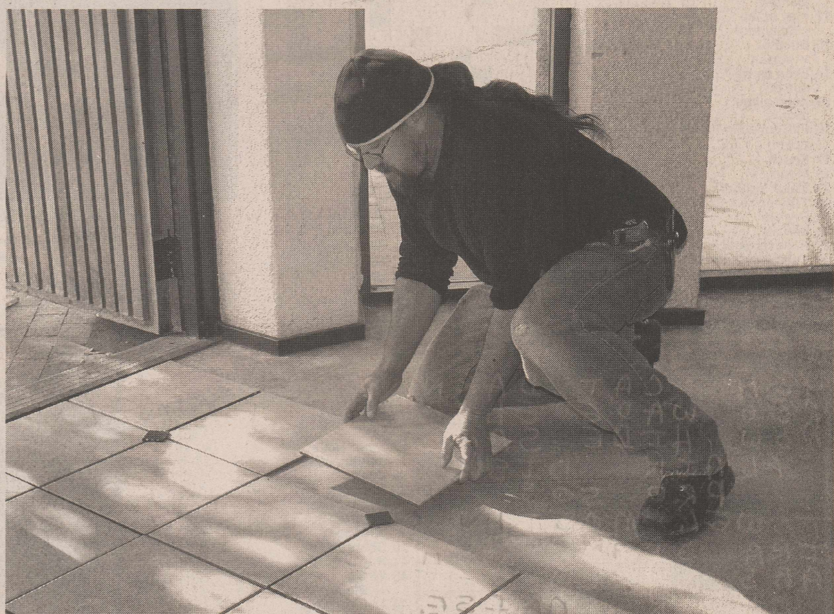
The new Visitor and Conference Center on the campus of WTC is getting new tile among other renovations that have been going on since the college acquired the building at the end of January from 37th Street Church of Christ. Carpet and new lighting are scheduled next with the remodeling of the kitchen and paint to follow. "The Center" will be rented out for public and corporate use as well as being the Visitor Center for the WTC campus. The building is anticipated to be ready for use in May. Above is Gary Antognini of Antognini Installations a Snyder business contracted by WTC.
