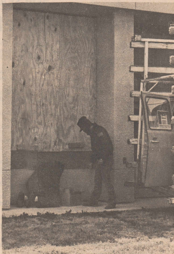
WHAT A PANE!—A large window on the Baptist Student Union is replaced following gale-force gusts on campus late last week. —James Hernandez photo
