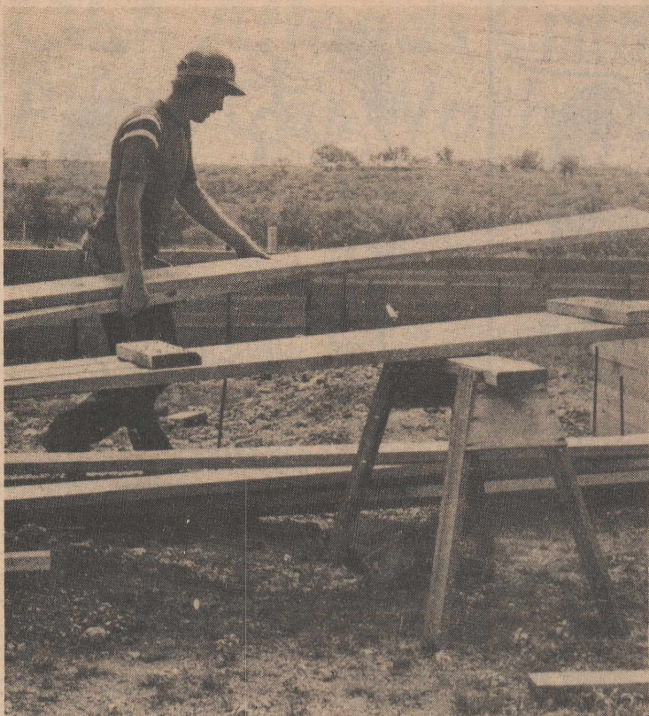
NEW PROGRAM IN PROGRESS — Residential Construction program student, Steve Fisher is busy on the job. The students are constructing apartments to be used for housing on the southeast corner of the campus. (photo by Debbie Sutton)
