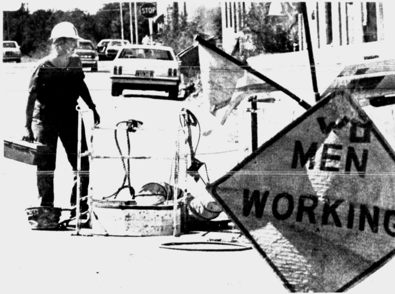
WORKING — Southwestern Bell cable splice technician Debbie Alford updated her "Men Working" sign to something more appropriate as she installed new underground cable recently adjacent to the post office. (SDN Staff Photo by Bob Campbell)
