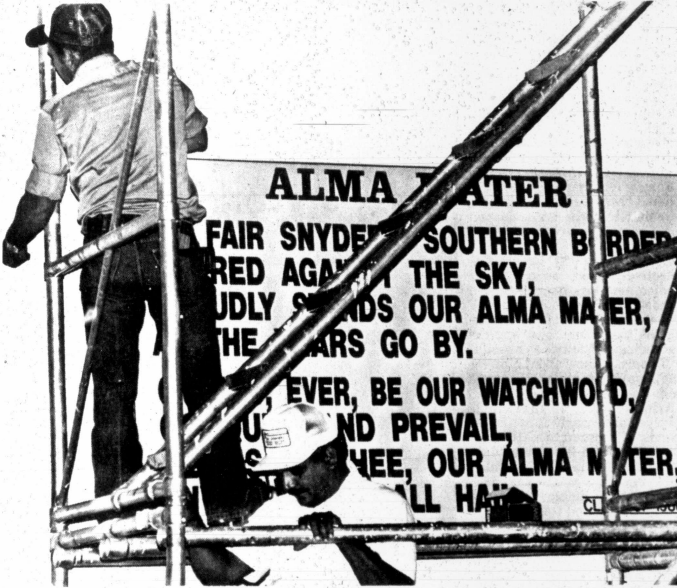
ALMA MATER - School maintenance men Don Compton, top left, and Juan Hernandez Friday morning erected the new school song sign that the
