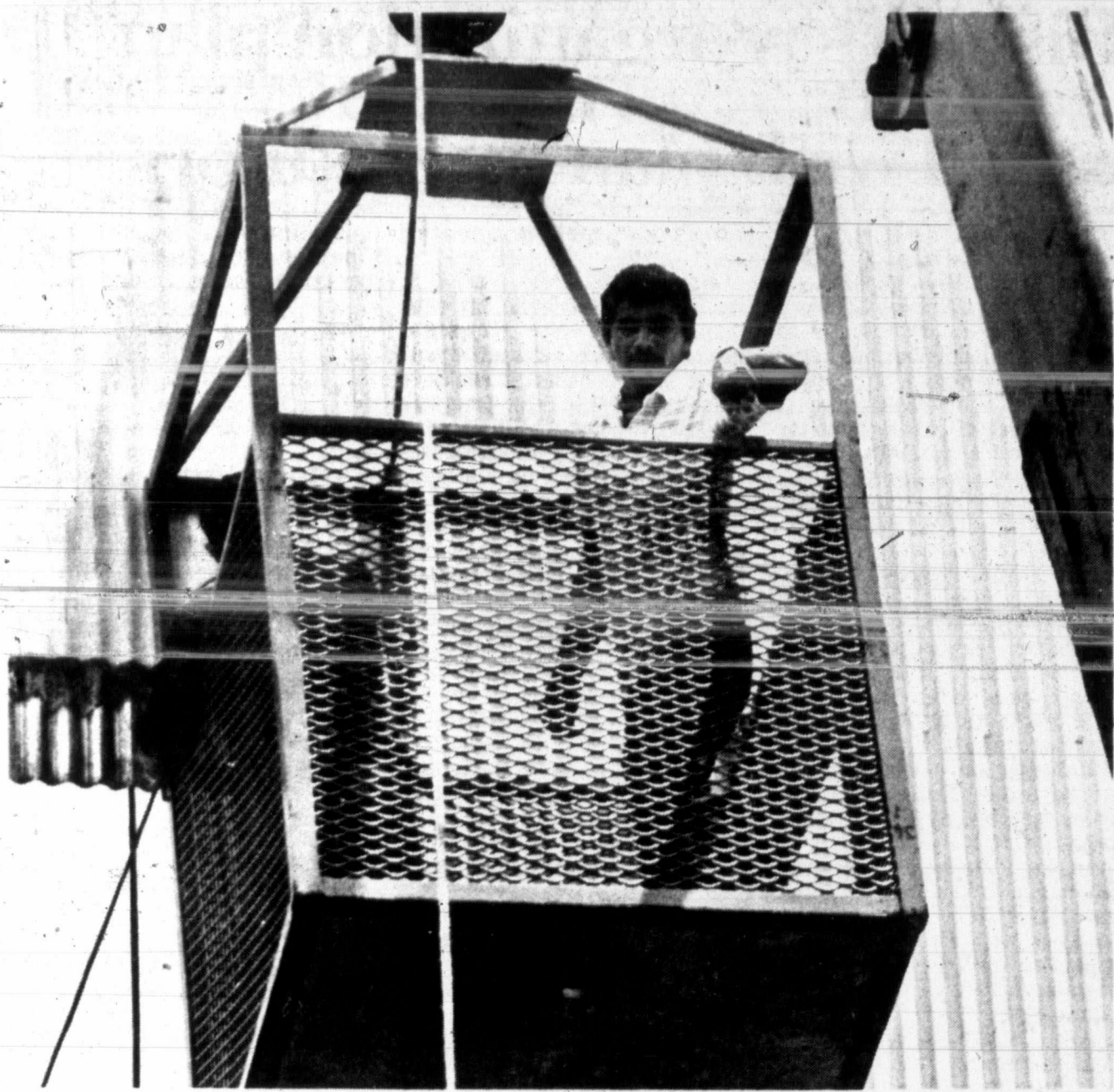
ELEVATED — Workmen last week were about 40 feet off the ground in a construction workers' bucket, dismantling the screen at the old Tiger Drive-in to make way for the new Wal-Mart store that will be built on the site. (SDN Staff Photo)
