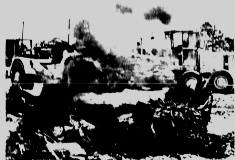
HEAT — Heat waves from burning debris distort the image of construction workers clearing property on the site of the old Tiger Drive-in theater in the 4500 Block of College Ave. Dirt work is continuing for the construction of a new Wal-Mart store at the location. (SDN Staff Photo)
