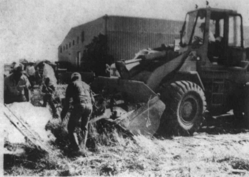
IN PREPARATION — When word was received of the Oct. 7 visit of a three-member team from the Texas Department of Corrections, local Industrial Foundation board members organized a joint effort to clean up the foundation-maintained Wickes Building. The building and other selected sites around Scurry County were stops on the group's visit. Their appearance here was part of statewide on-site inspections of cities and counties applying for prison projects. (SDN Staff Photo)
