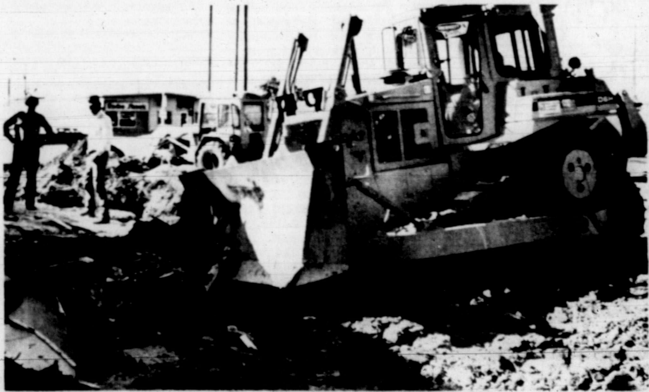
COMING DOWN — A Grimmitt Brothers bulldozer Wednesday afternoon moves in to raze the foundation of the Southside 66 station at 3800 College Ave., where a new Phillips 66 convenience
