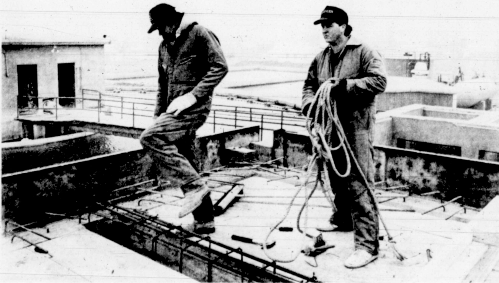
CHILLY WORK — Joseph Cabrera, left, and Toby Roemer are among the workers involved in the construction of a rapid mix basin at the city water treatment plant on Ave. M. Work was underway Wednesday afternoon with temperatures in the 30s and a stiff northern wind. The project has been contracted to Decker Construction Co. of Abilene. (SDN Staff Photo)
