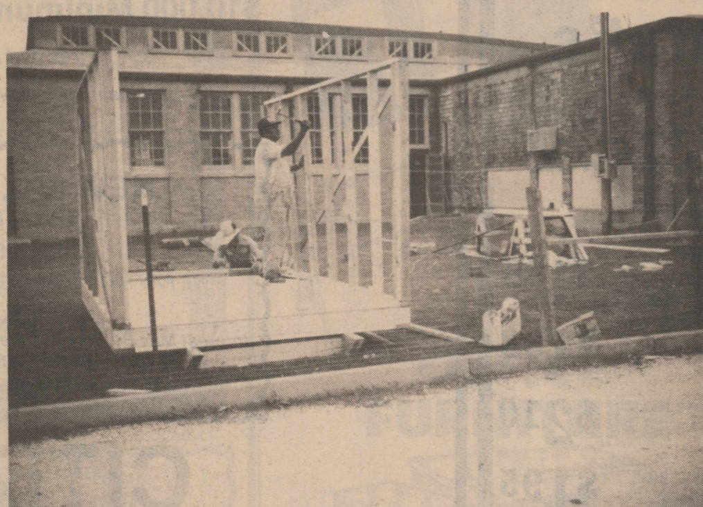
A HAPPY SIGHT for Knox City residents is the evidence of the actual construction which has begun on the conversion of the elementary gym into a modern auditorium, long needed by the entire community. A fence has been built around the work area and workers, including Leo Harris, in foreground, were busy Tuesday morning constructing a tool shed for the project tentatively scheduled for completion in August. Larry Dennis of Rule is contractor.
