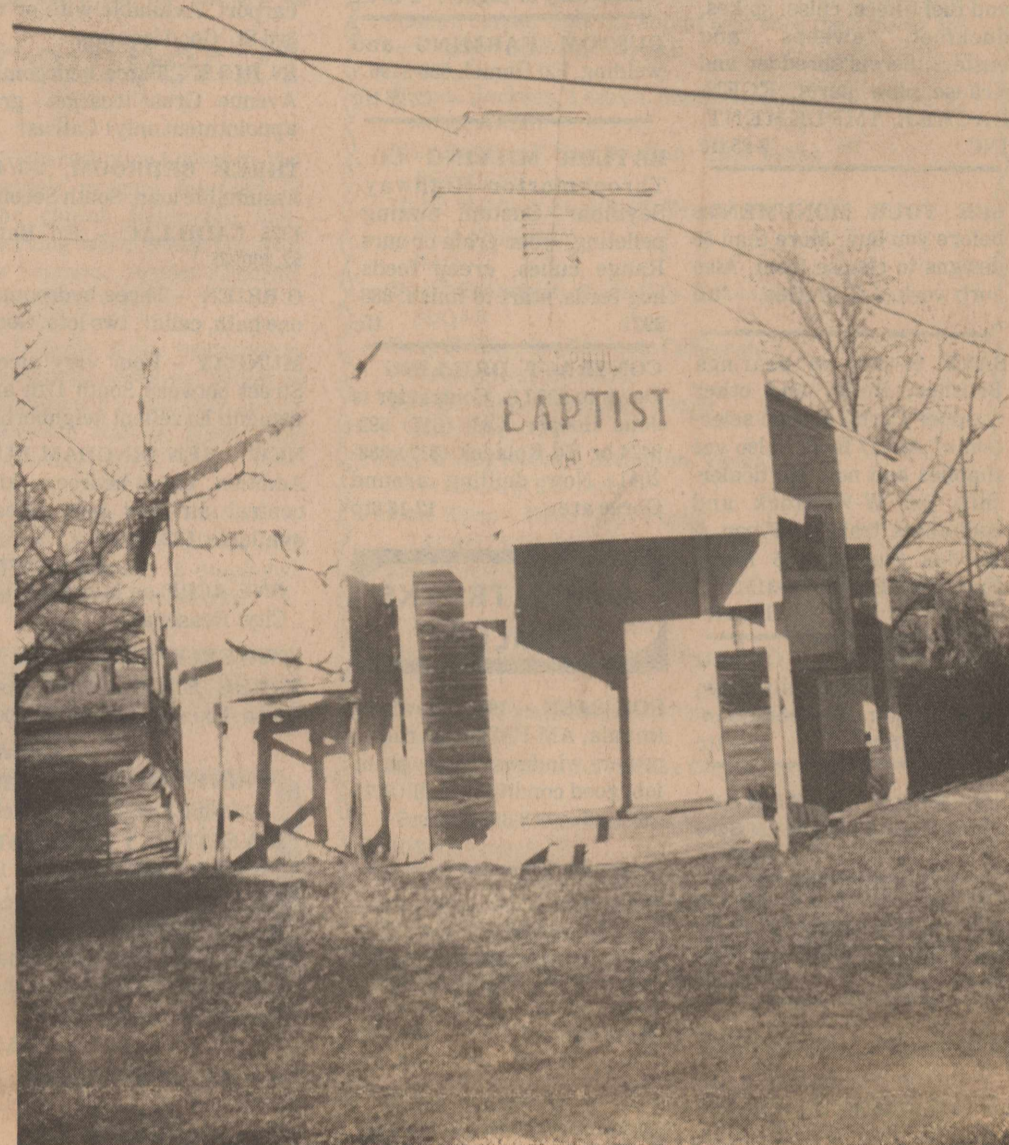
MEMBERS OF St. Paul Baptist Church recently have begun a remodeling program. As noted in the above picture, the exterior shingles are being removed for an addition across the church's front. Also a complete renovation of the interior will be done.
