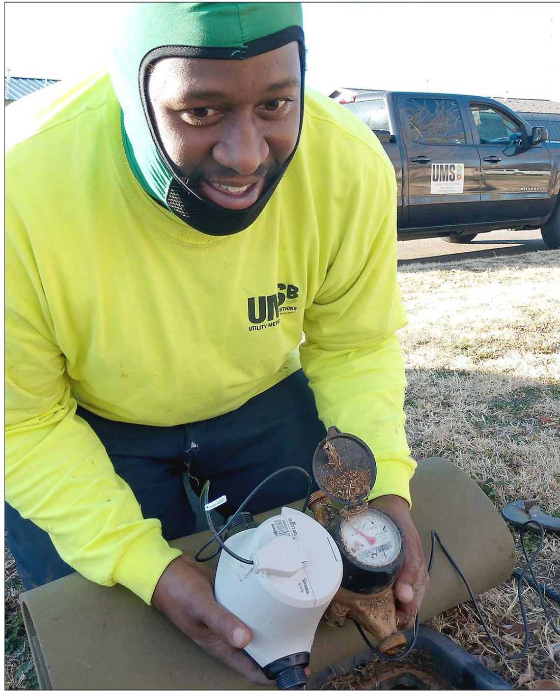
Joshua Garrett of Charlotte, North Carolina, replaces an old water meter (right) with a new electronic meter (left). Garrett and several other employees of UMS are in town to replace all of the city's water meters as part of a larger infrastructure upgrade project.
