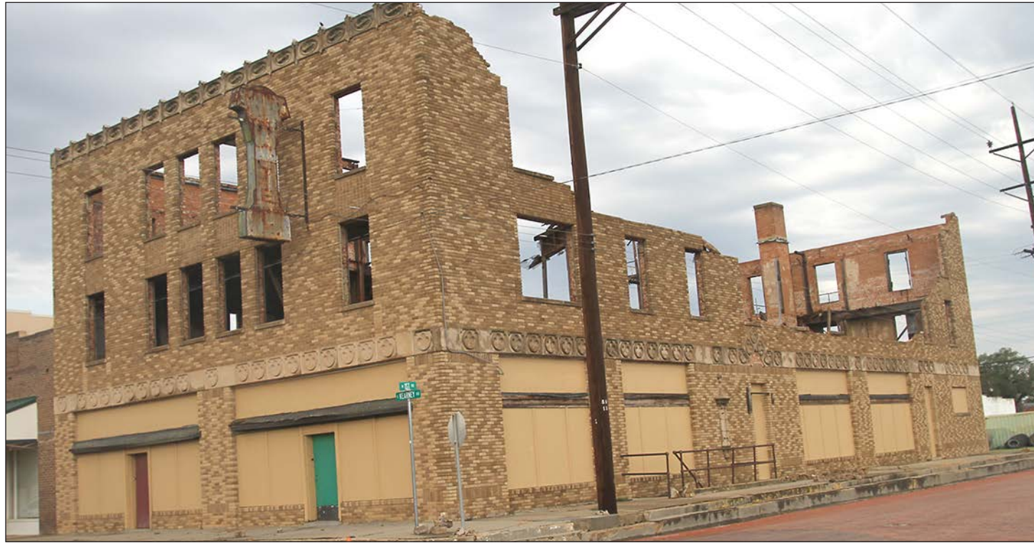
The old Antro Hotel suffered severe damage when a storm struck the city Sunday night. See more photos on page 8. ENTERPRISE PHOTO
