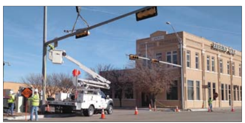
Drive safe Workers take down the old traffic signals at US 287 and Kearney last week as the installation of new signals progresses. Drivers are urged to use extreme caution as there will be no signals to stop highway traffic until the project is completed.
