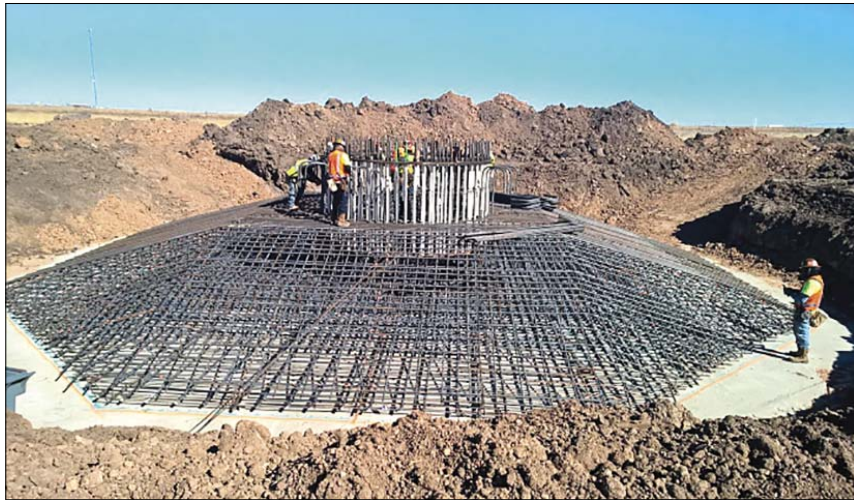
Workers position reinforcing steel as part of foundation work at a turbine site on the Salt Fork I Wind Energy Project in northwestern Donley County recently.
