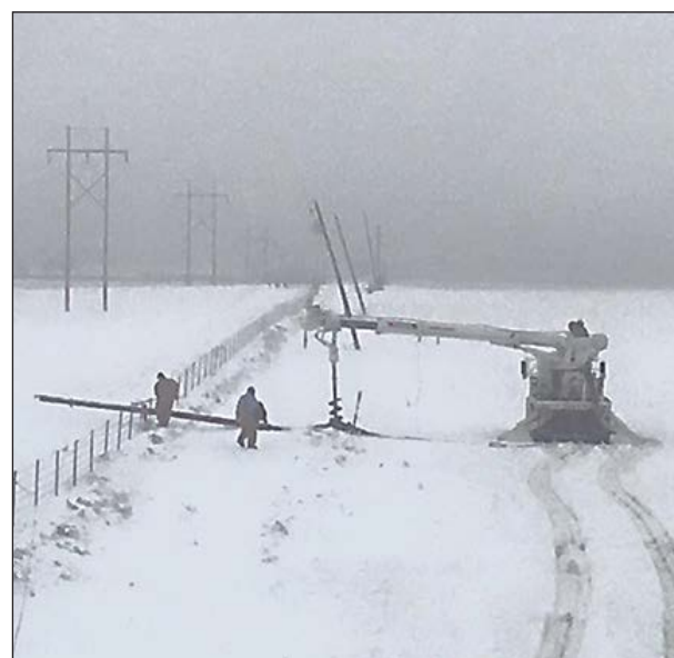
A Greenbelt Electric crew replaces broken poles on the McDowell Ranch near Shamrock. The cooperative lost 250 poles in the storm.
