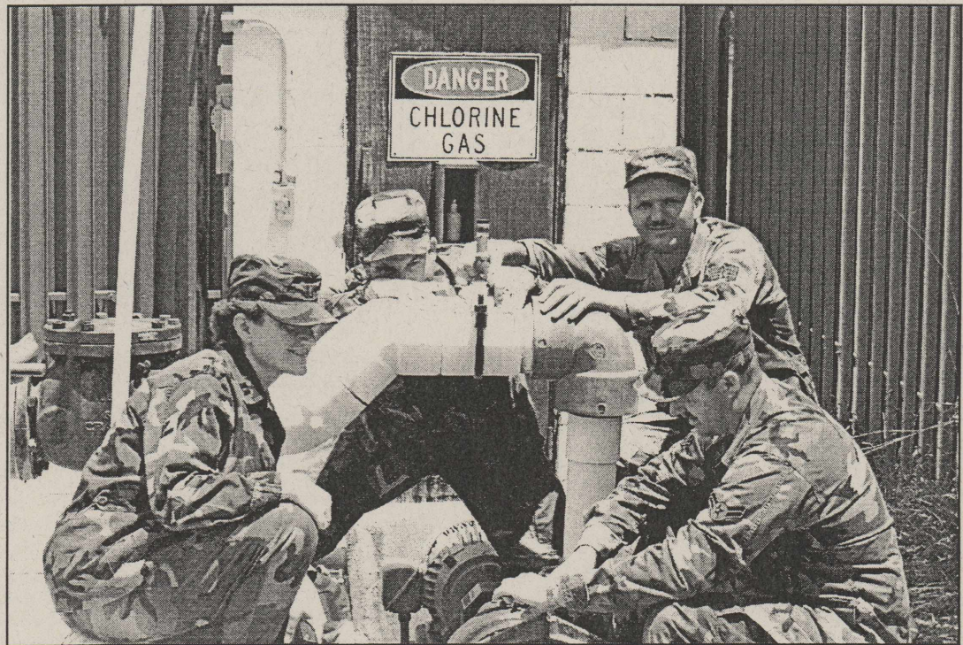
Capt. Anne Coverston, commander of the 64th Civil Engineer Squadron operations flight, and three members of her staff check the chlorine filter at Reese Beach, Reese Air Force Base's swimming pool. The members are, from top left, Staff Sgts. Jeff McKenzie and Kevin Johnson and Airman 1st Class James Frazier.
