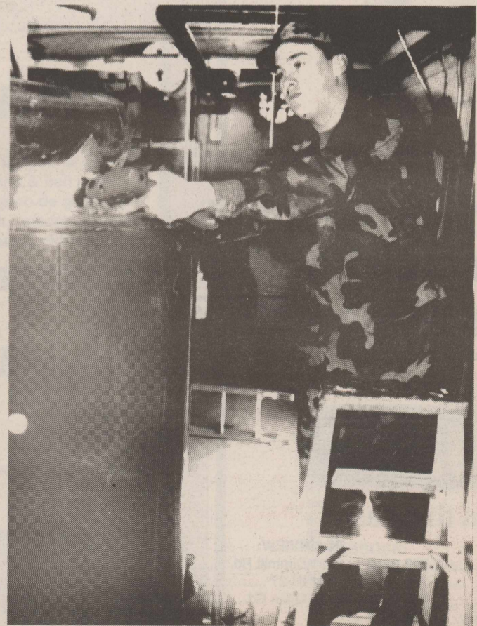
Airman 1st Class Keith Morgan replaces a vent on the waterheater at the fitness center.
