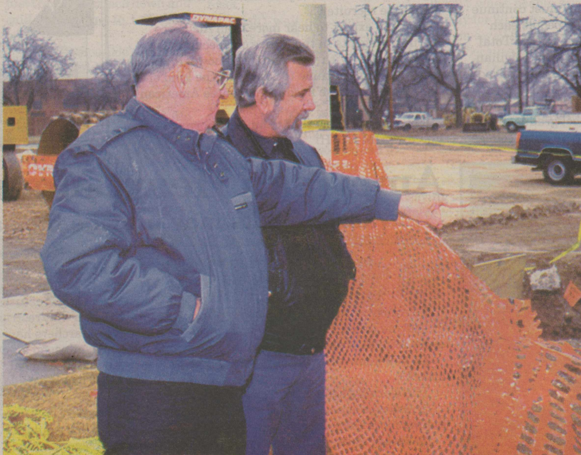
Chuck Gerrior and John Hateway conduct a ground safety inspection on a construction site here.
