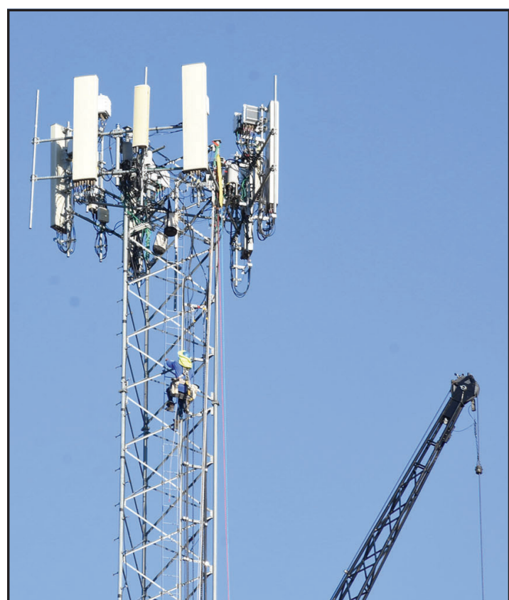
A crew has been working the past couple of weeks installing upgrades on the cell tower at Reeve Lake. Unfortunately, some AT&T and other phone customers were without service for a couple of days. The work crew had their meals delivered via a "rope elevator" each day.
