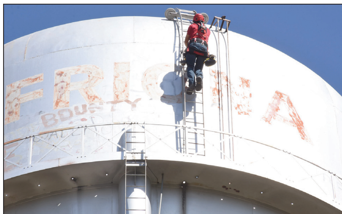
Oscar Ostos, an engineer with Hi-Plains Civil Engineers, climbed the north water tower on Wednesday to perform a structural inspection and take paint samples. Oscar is the engineer for the City of Friona. Plans are to repaint the tower as a cheeseburger. More details next week.
