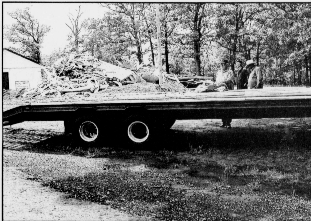
OUT WITH THE OLD AND IN WITH THE NEW-The old Maple Springs Church building was reduced to a pile of rubble this week as the church prepares to build a new fellowship hall. The workers who have helped to tear down the building are appreciated. Watching the dozer, operated by Chad Parish, work were Charlie Young, Jesse Brown and Scooter Parish. (Staff Photo Nancy Brown)
