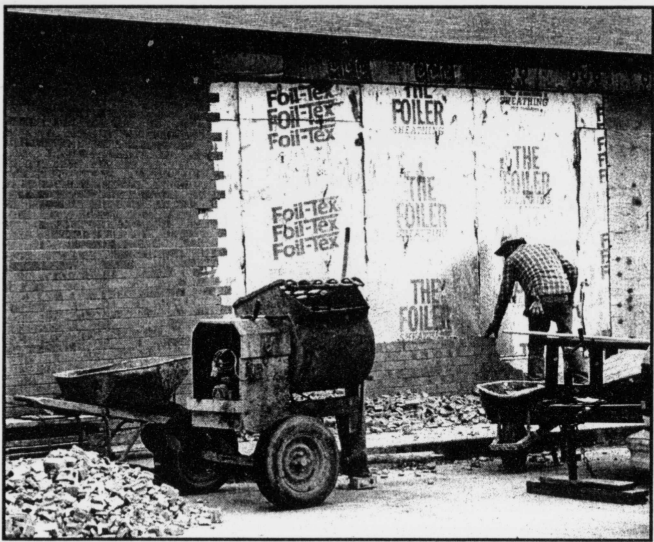
REPAIRS-The Bogata Post Office received repair work last week to the wall that was damaged when a vehicle accidentally hit it recently. It is now good as new. (Staff Photo Nancy Brown)
