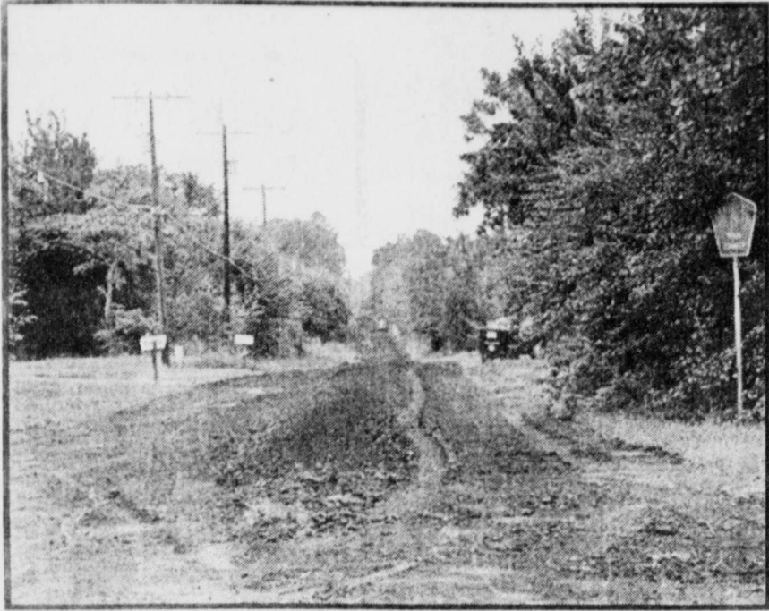
MAKING HAY AND ROAD REPAIRS -are usual summer time work and NW 5 (Crawford Lane) in Talco is receiving a work over. Other road repairs being made in the area are on the old Greenhill Road off FM 71 E at Meadows Curve. (Staff Photo Nancy Brown)
