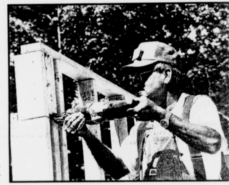
EDDY DENNY , member of the First Baptist Church of Bogata, works on a Texas Baptist Men Retiree Builders construction project near Paris, building a home for an 11 year old girl and her family.
